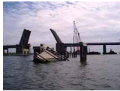
Wrecked Highway 90 Bridge at the mouth of Biloxi Bay, following Hurricane Katrina in 2005.
